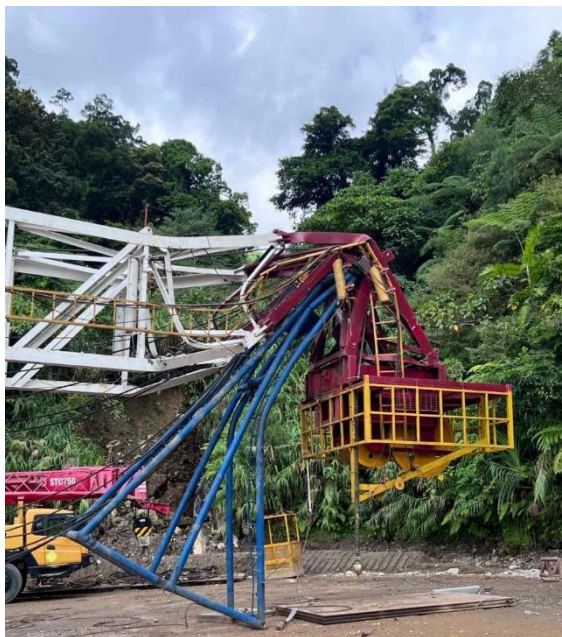
Left: Result of the raising wire failure.
